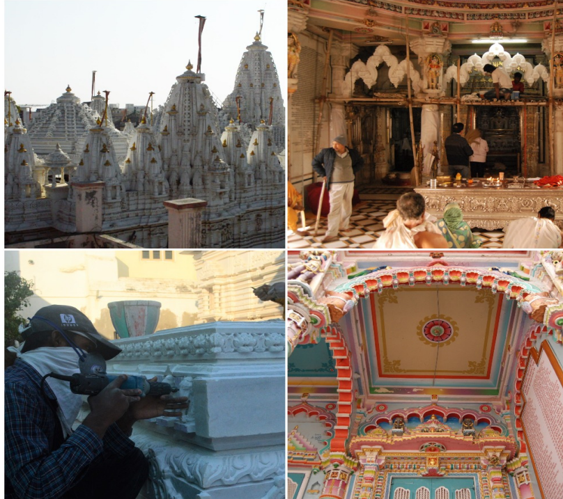
Figure 5.2. (clockwise from the top left) Exterior of the Sri Panchasara Derasar; Interior Renovation at the Derasar; Style of a Newer Jain Temple; and Construction of a New Jain Temple.
